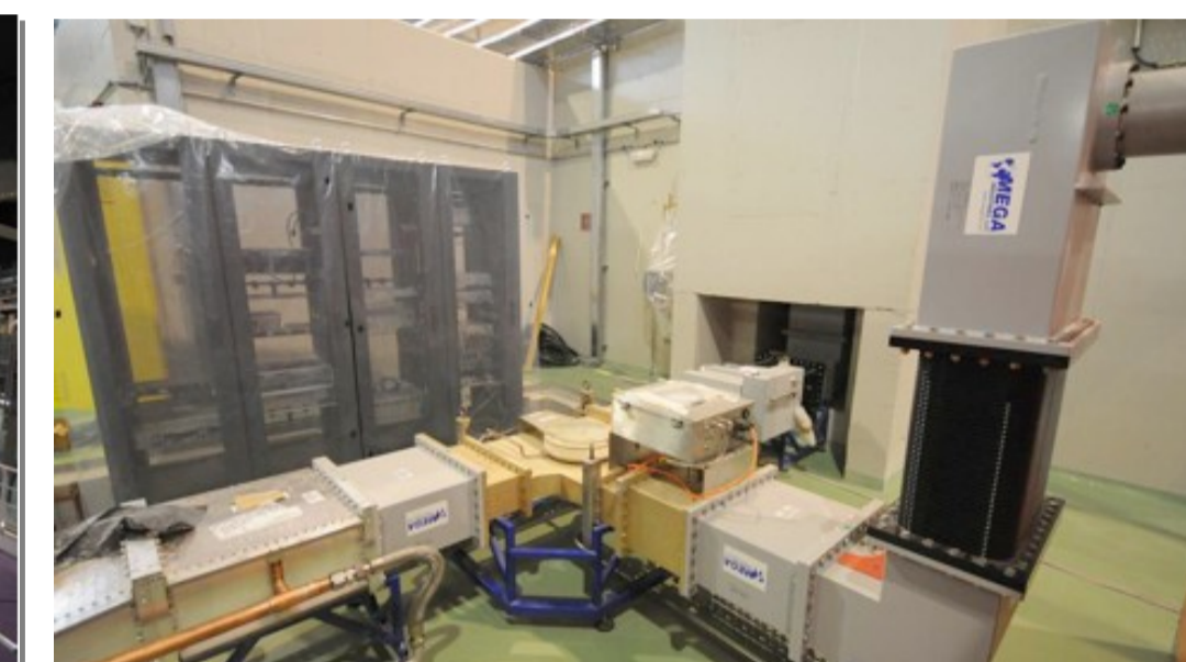
Up: Waveguide of the booster RF. Down Booster RF cavity
